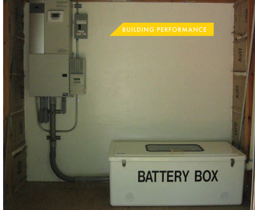
Solar power management system and battery storage.
