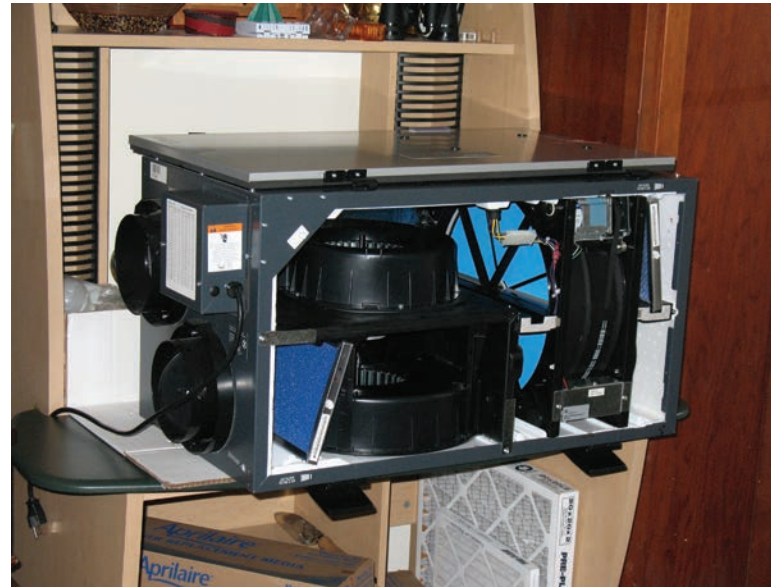
This Venmar DUO 1.2 ERV photo was taken before I moved it to the crawl space and connected it to the ERV ducts that are located there.
