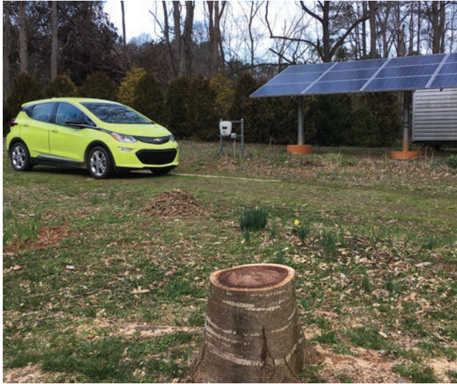
Grandchildren's Mimosa stump, pole mount PV, backup batteries, controls, and automatic power transfer building, Bolt EV, and level 2 home charging station.
